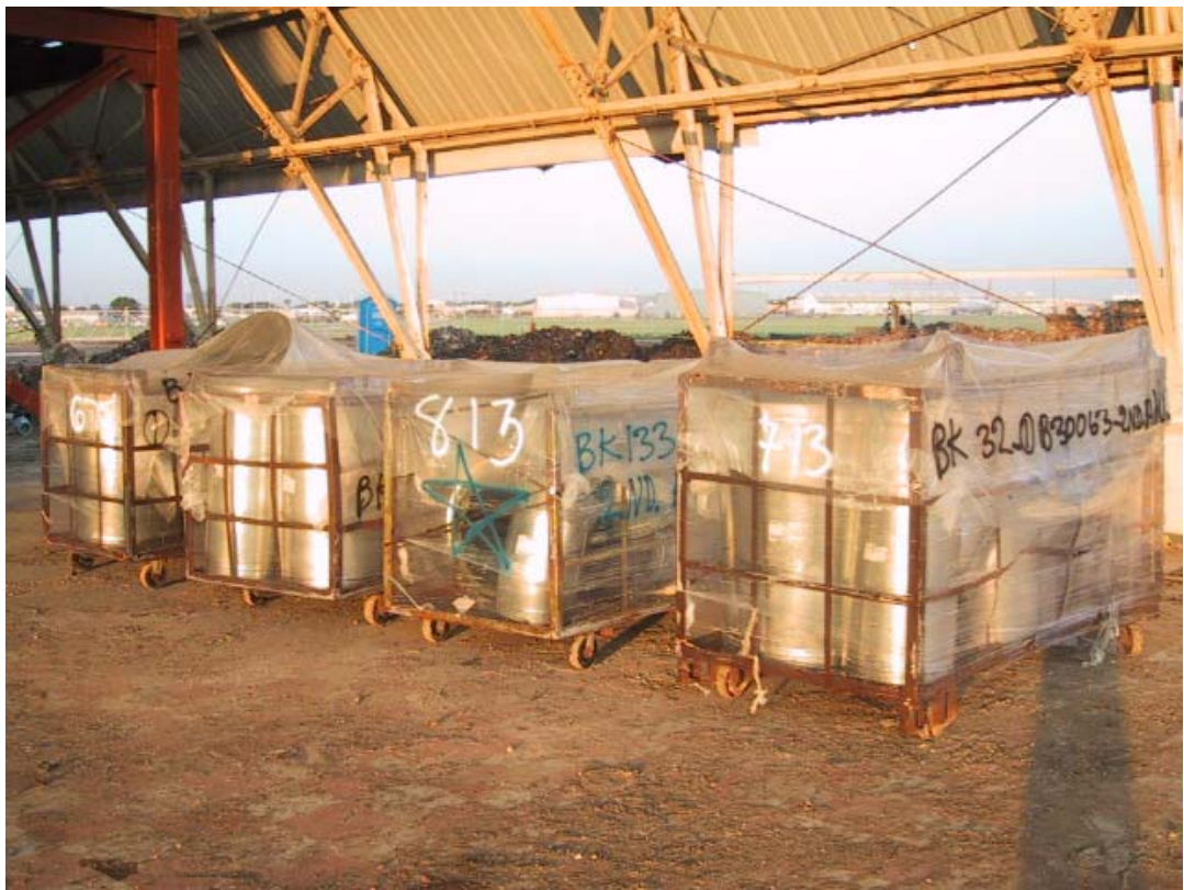
HVAC duct work delivered and ready for install
