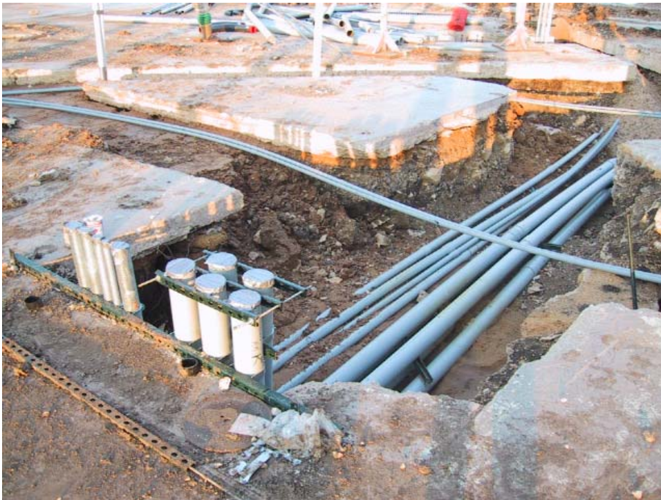
Electrical power stubbed into mechanical room
