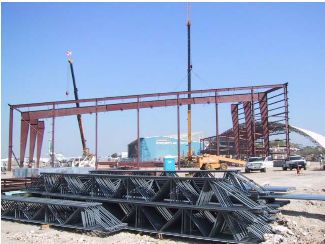
Main exhibit hangar steel finally going up – View looking North at what will be windowed end of hangar
