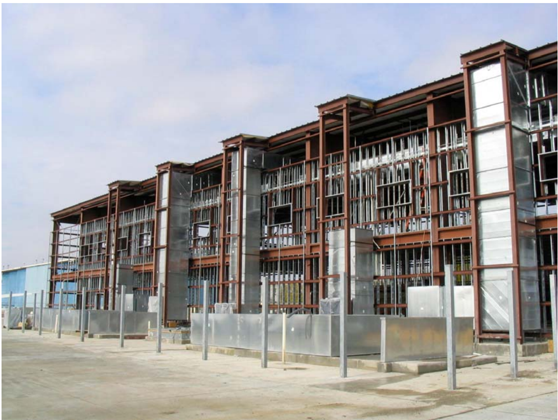
Exterior HVAC ducting on main hangar
